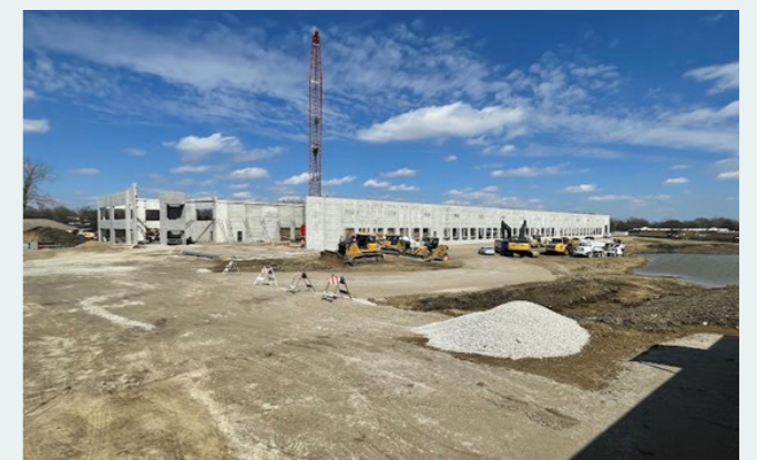
Quick progress has been made as tilt slab construction commences in West Chicago
