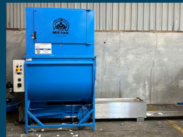
Polystyrene Compactor, Mainfreight 2Home Christchurch
