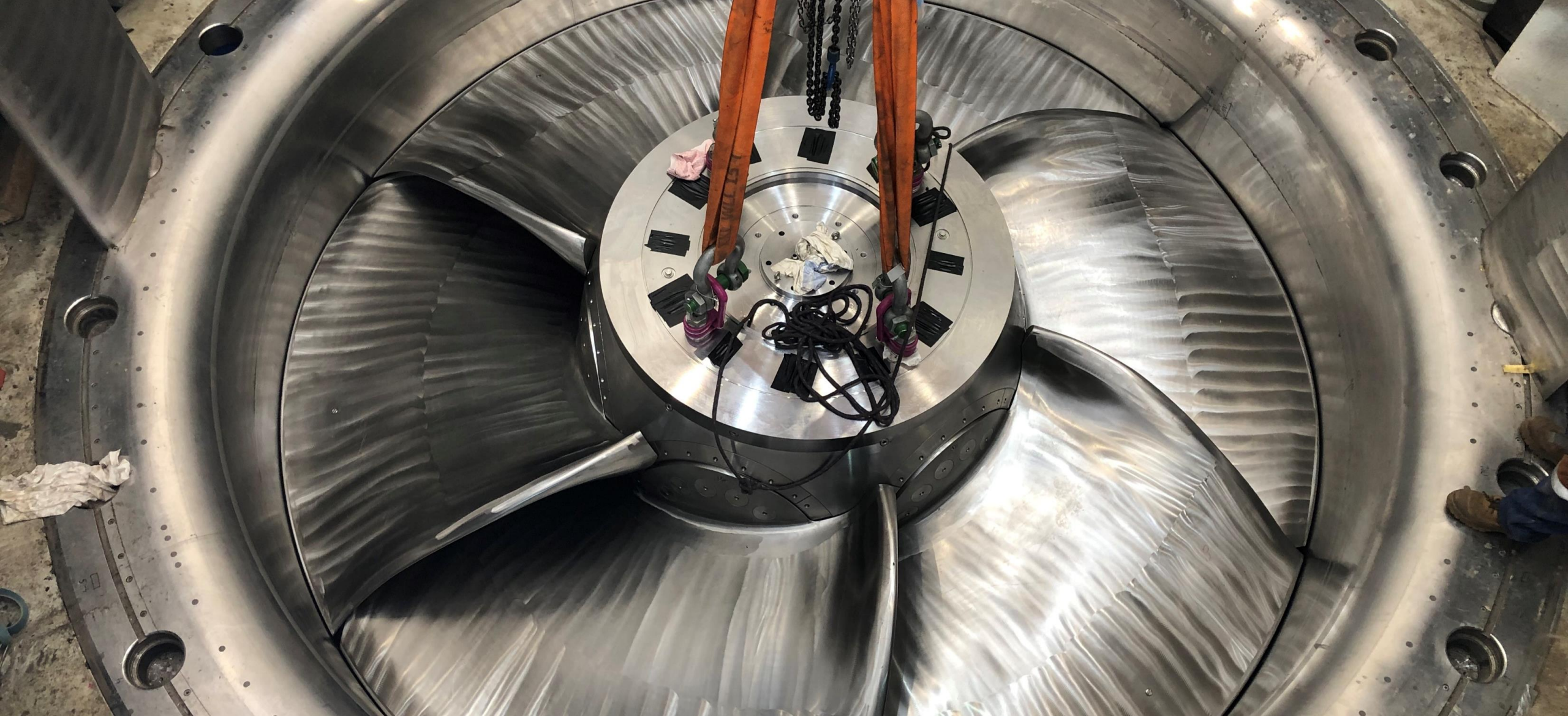
Karapiro Hydro Turbine
