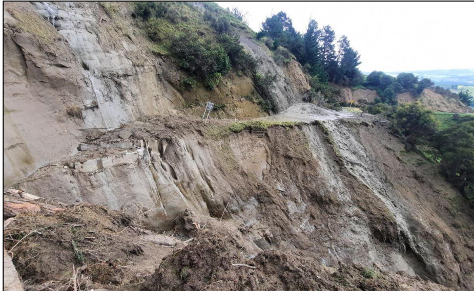
Road washout near Tutira.
