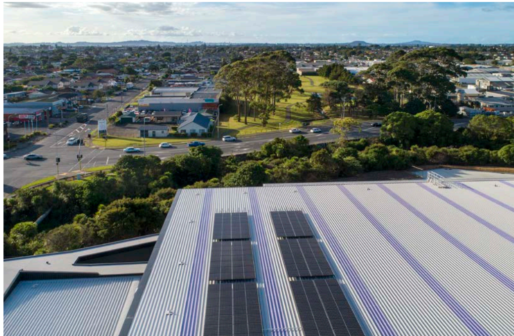
Dicker Data roof-top solar panels, M20 Business Park, Manukau
