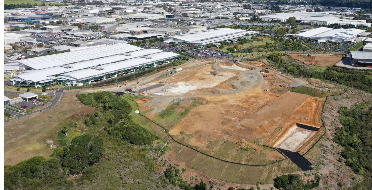
Ground works progressing well on the fifth R&D and manufacturing facility in Auckland, New Zealand.
