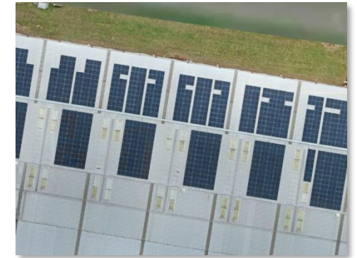
Laminex® Toolara (Australia) have started generation from their new roof solar installation
