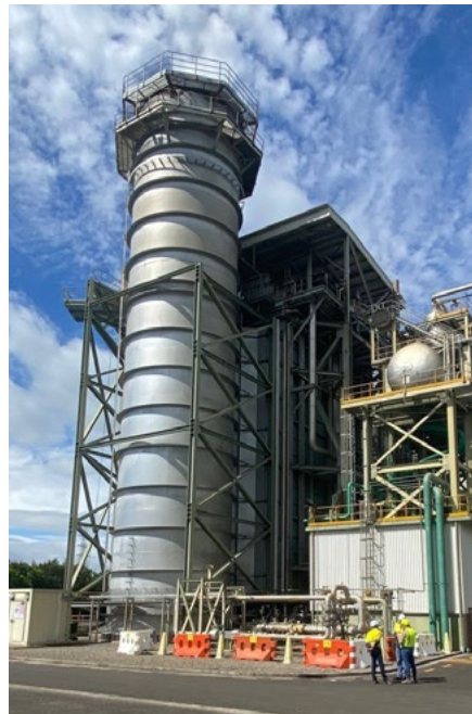
TCC's Heat Recovery Steam Generator at Stratford.
