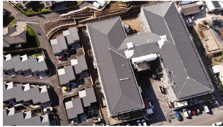
An aerial view of the new care centre at Lauriston Park being constructed.
