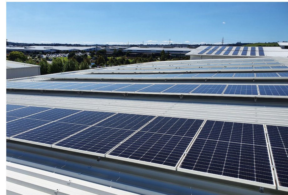
Solar at PMA, Highbrook Business Park
