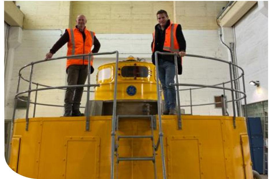
Stephen Fraser (GM Generation) and David Prentice (CE) at the newly commissioned Waipori 4 station generator
