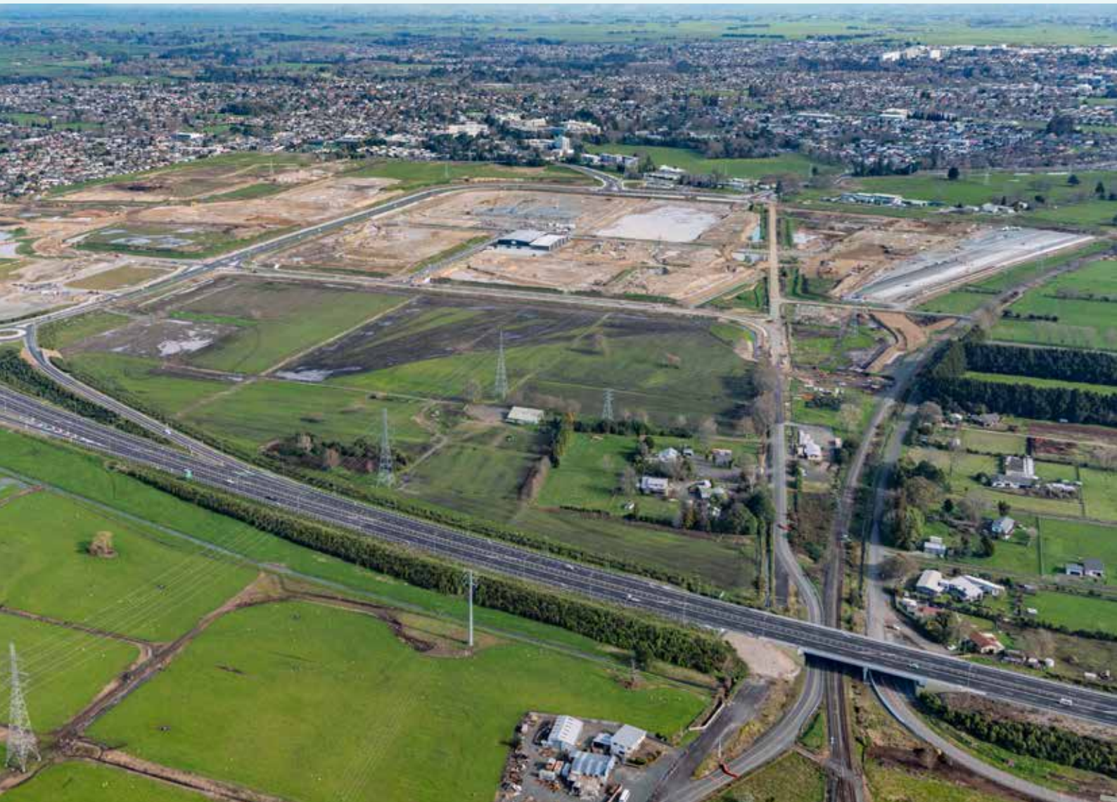
Above, progress of the Ruakura Superhub under development in Hamilton, with the inland port at the far right of the earthworks and the Waikato Expressway in the foreground. Below, the pavement of the inland port, and the East Coast Main Trunk rail line, can be seen on the left of the picture.
