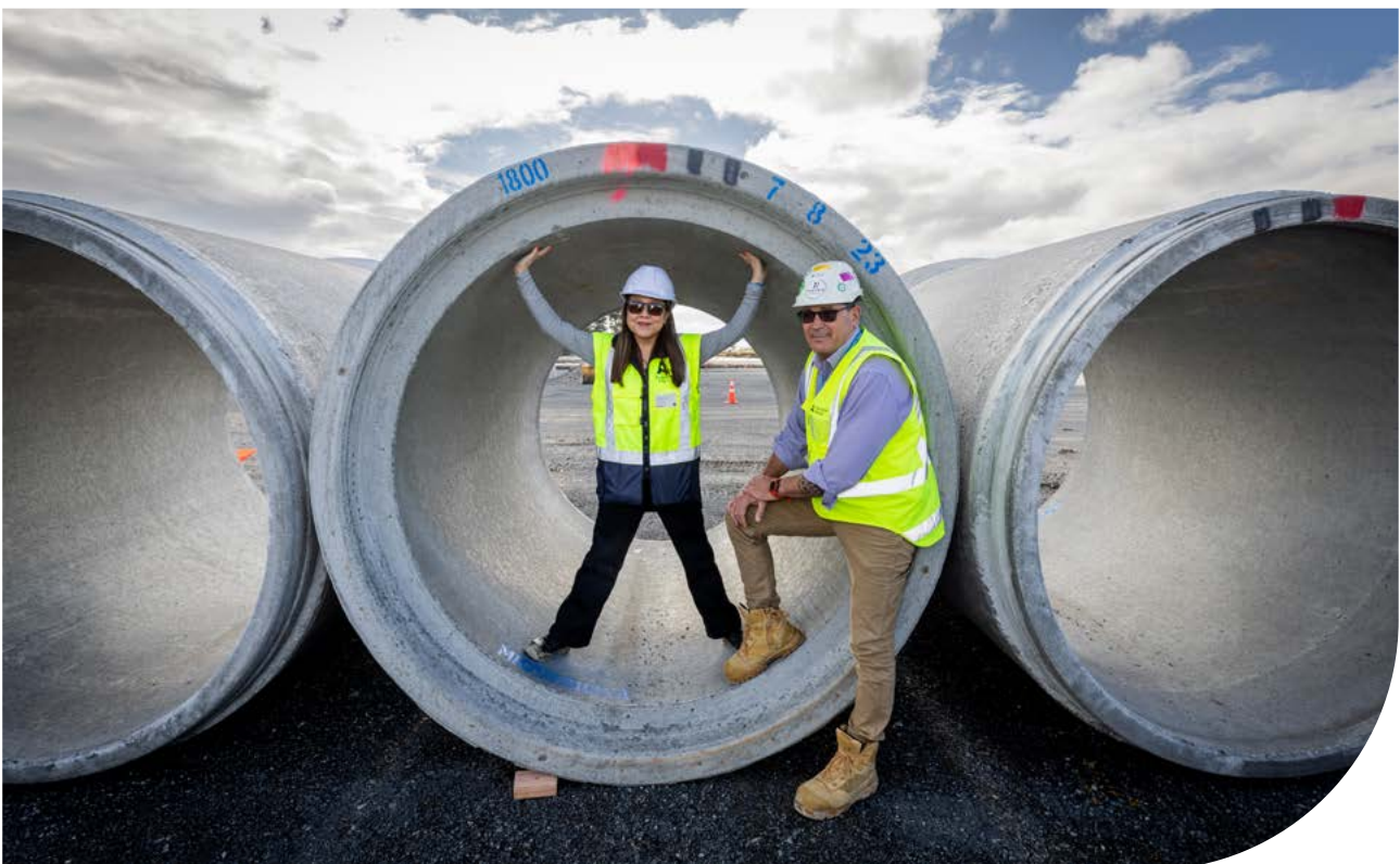
Pre-implementation Programme Manager Adrienne Khor and Mark Blanchard, Construction Operations Manager, demonstrate the size of stormwater pipes installed as part of a 3.5km network.
