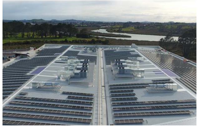
2 Mānawa Bay will have what is believed to be the largest rooftop solar array in New Zealand.
