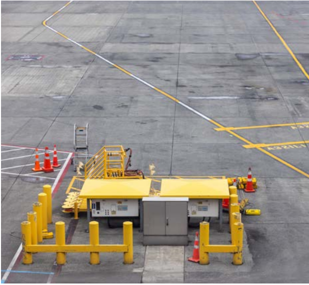
3 Ground power units enabling international aircraft to connect to NZ's low-carbon electricity supply.
