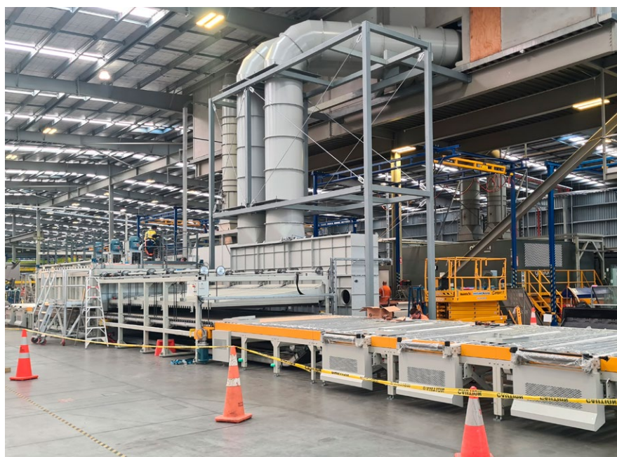
New furnace at Highbrook plant in Auckland, New Zealand
