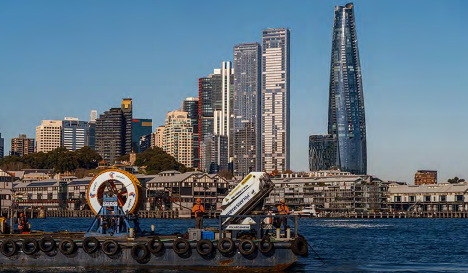
Pictured: Installation of a new fibre optic cable across Sydney Harbour, as part of Telstra InfraCo's InterCity Fibre Network build, NSW
