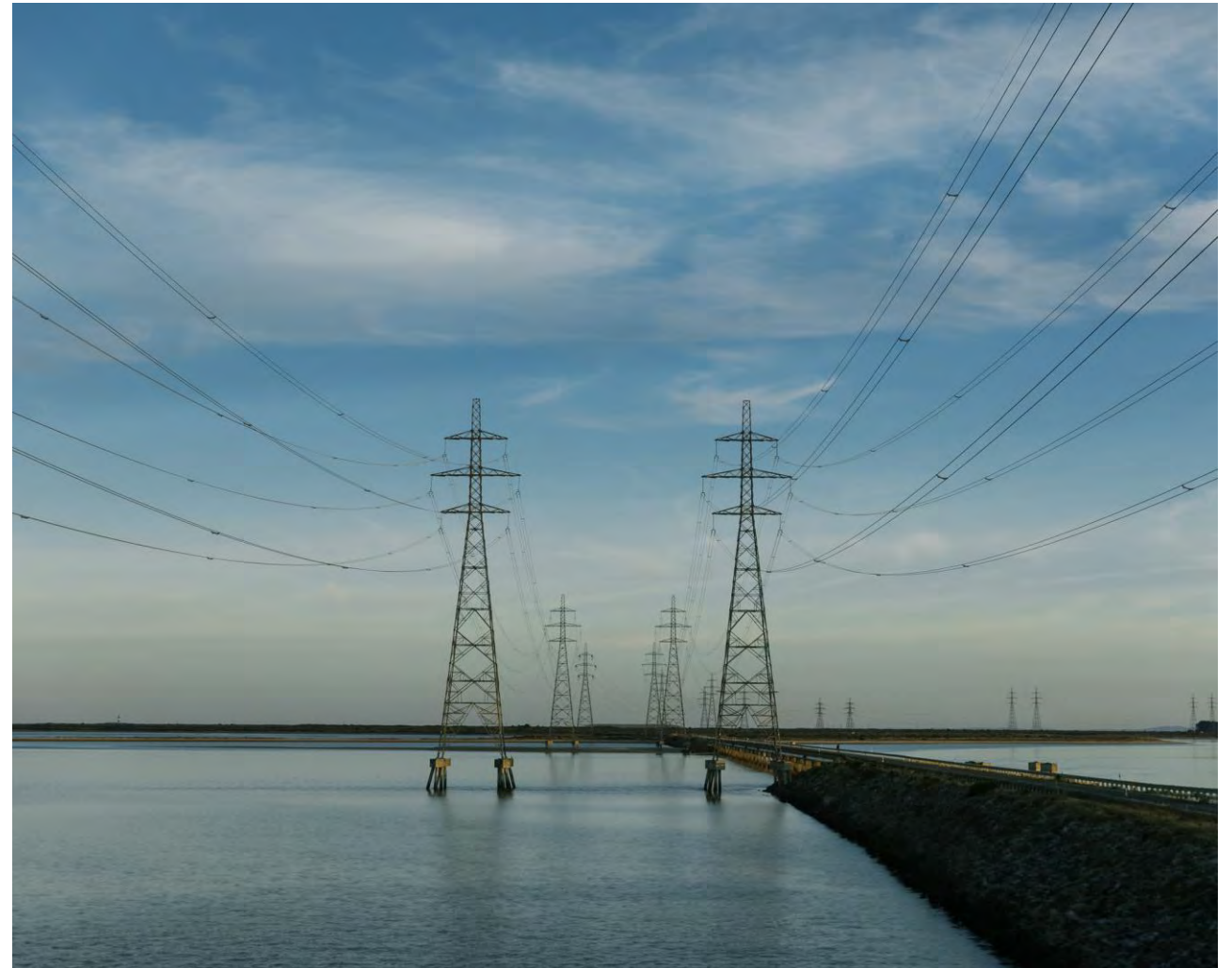
Transmission lines near New Zealand's Aluminium Smelter in Southland
