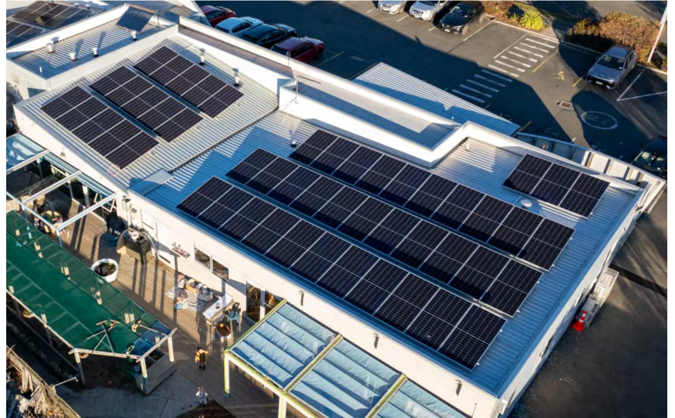
Solar installation at Waipuna Community Services in Canterbury
