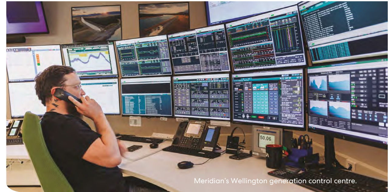
Waitaki Power Station control room.
