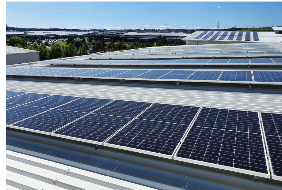
PMA, Highbrook Business Park, solar panels installed on existing property
