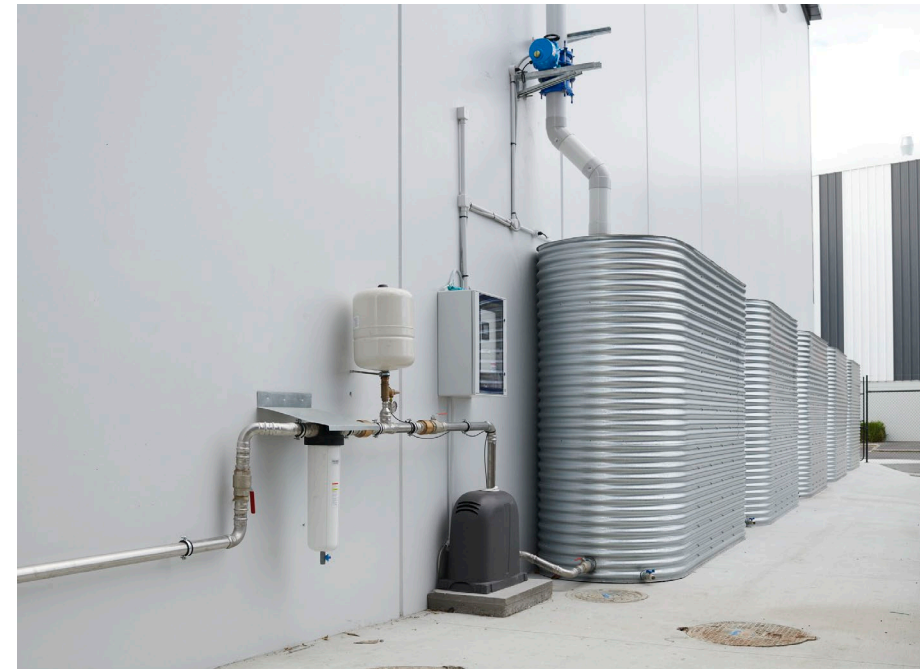
M20 Business Park – Rainwater harvesting
